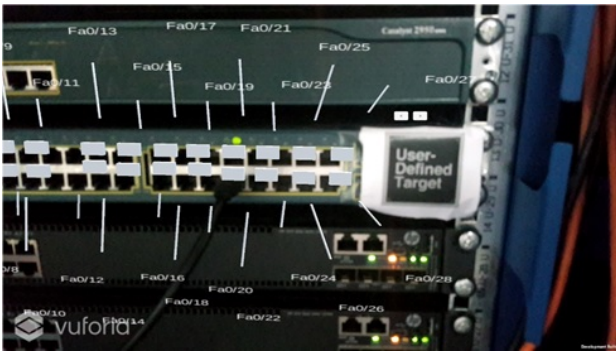
Fig. 4. An example of the overlaid network switch information.
